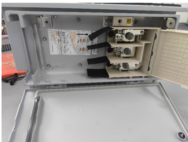
AC side terminal block
